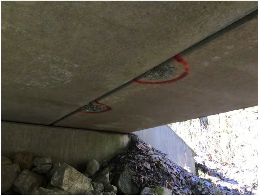
Damage to underside of slabs
